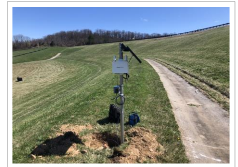
Installation of telemetry datalogger unit at Dike
