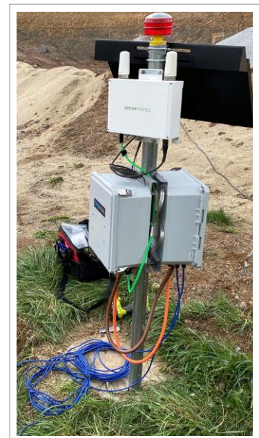
VWPs grouted and buried in newly constructed sand drain. Cabling run back to a central datalogger location
