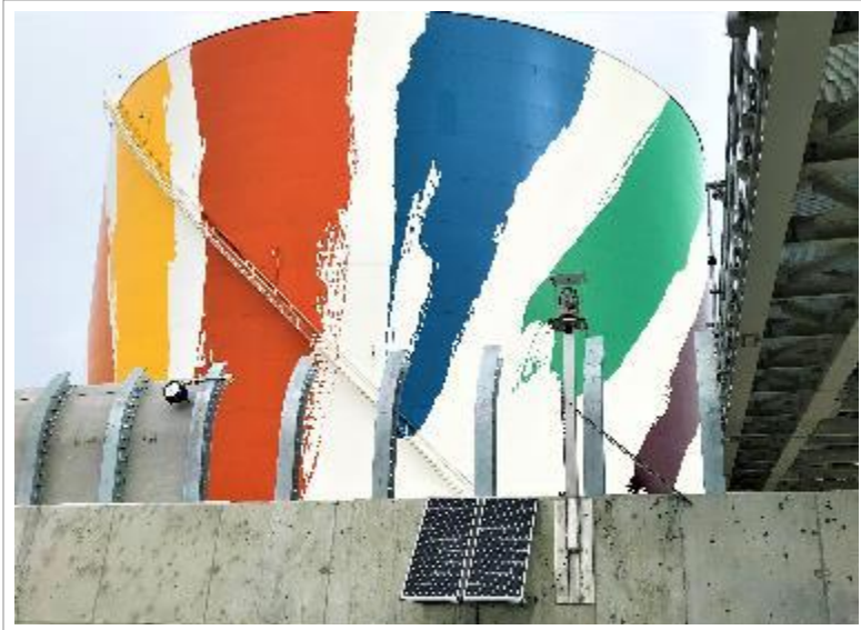
Automated Motorized Total Station (AMTS) surveys LNG tank for settlement every two hours during construction, at costs significantly less than weekly survey crew
